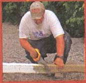
Carl Grant, Jr. Tiler Red Seal journeyman carpenter and lead hand, Company: Joldama Renovations, Ottawa, Ontario (Photo by M. Heath, used with the permission of Carl Grant, Jr.)
